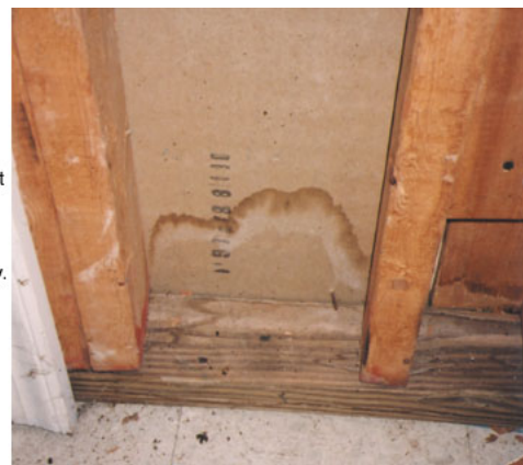
Water stain on a basement wall - locate and fix the source of the water promptly.
