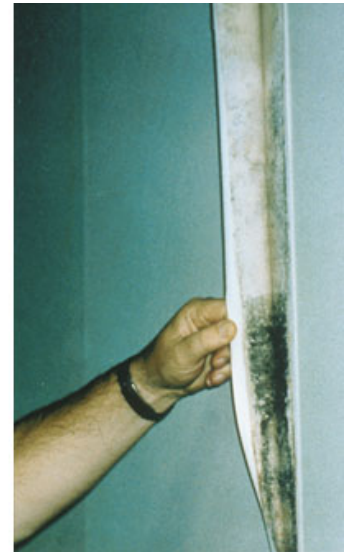
Mold growing on the back side of wallpaper.
