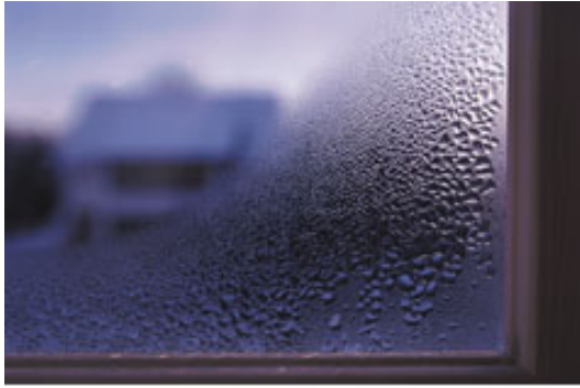
Condensation on the inside of a windowpane.
